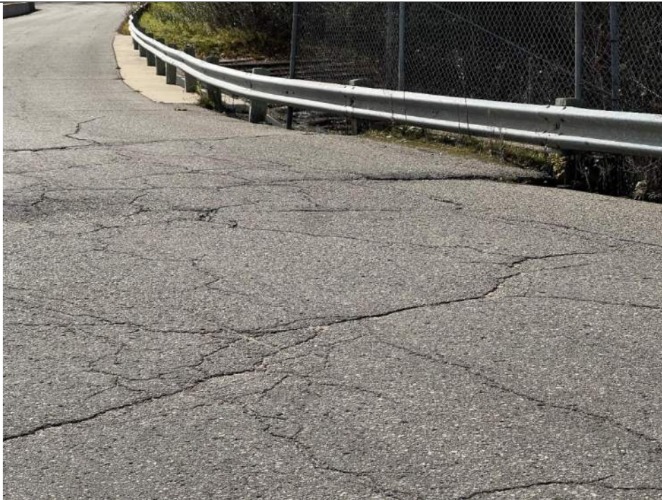
Photo No. 54 – Cracking of Pavement over Primary Spillway – Looking Left
