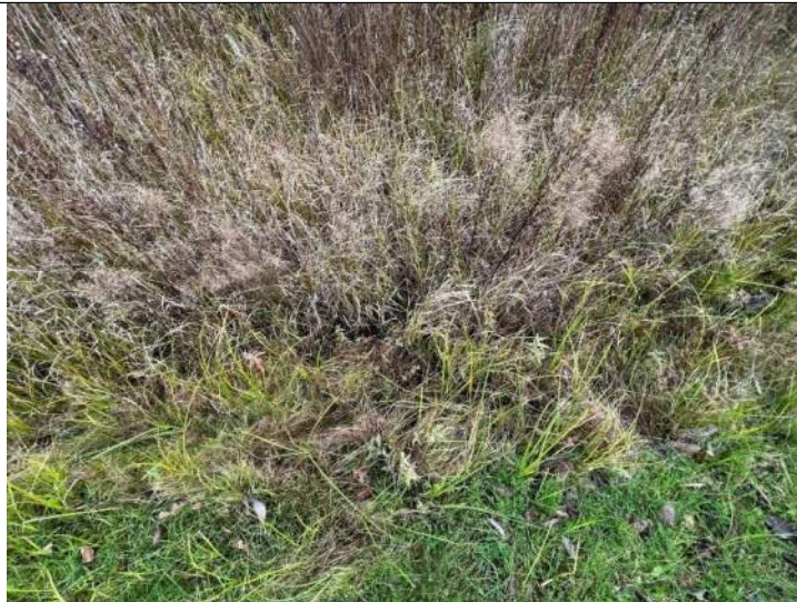
Photo No. 34 – Right Embankment – Downstream Toe Seepage
