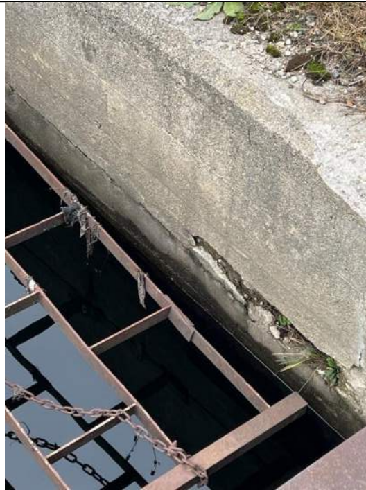
Photo No. 8 – Auxillary Spillway – Concrete Deterioration Right Wall
