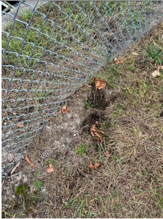
Photo No. 9 – Auxillary Spillway – Erosion at Fence
