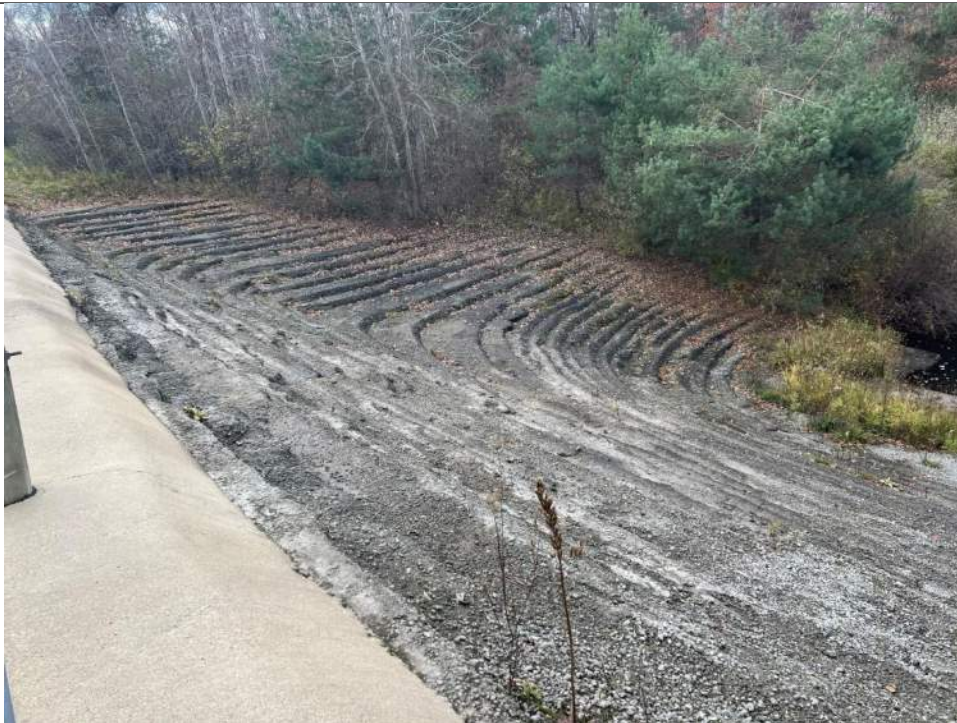
Photo No. 92 – Downstream Left Embankment RCC Slope Deterioration – Looking Left
