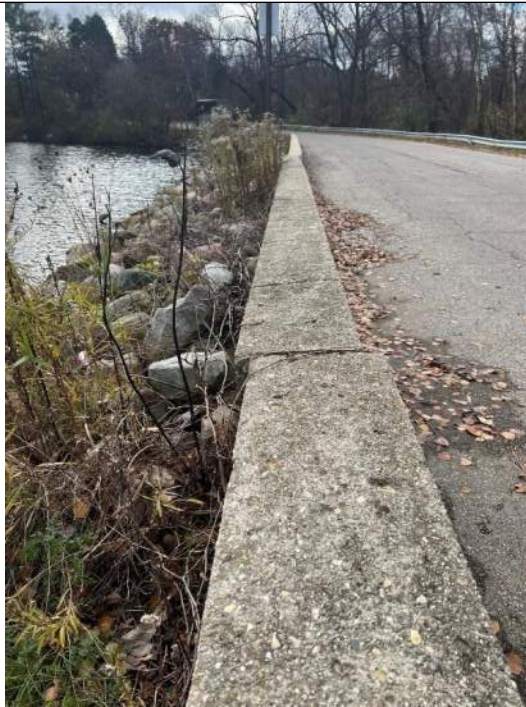
Photo No. 79 – Upstream Left Embankment Flood Wall Transition to Riprap and Wall Rotation - Looking Left
