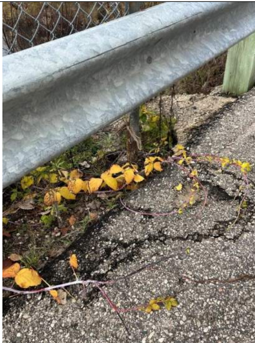
Photo No. 96 – Pavement Deterioration at Primary Spillway Downstream Side of Crest – Looking Downstream
