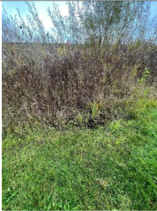
Photo No. 27 – Right Embankment – Downstream Toe Seepage
