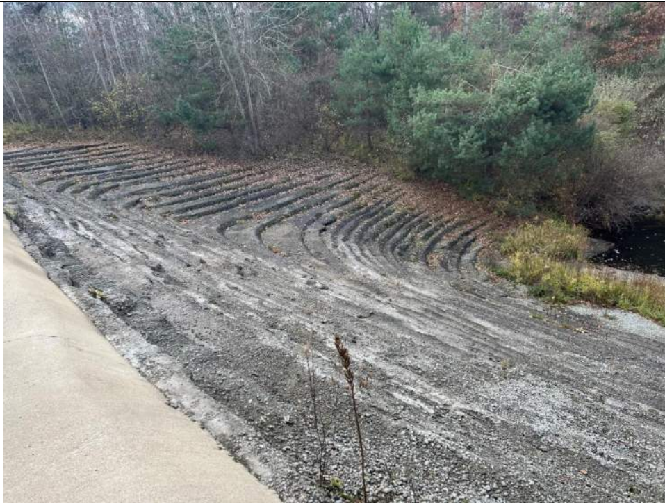
Photo No. 91 – Downstream Left Embankment RCC Slope Deterioration – Looking Left
