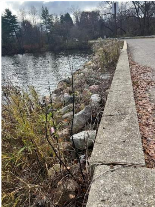
Photo No. 76 – Upstream Left Embankment Flood Wall Transition to Riprap and Wall Rotation - Looking Left
