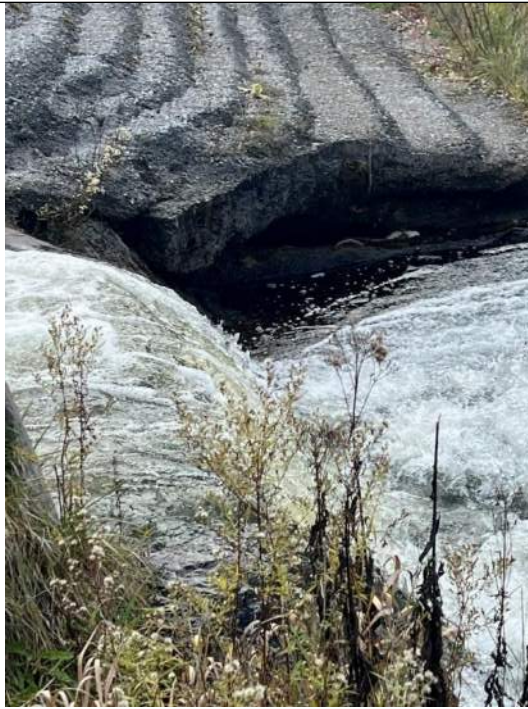
Photo No. 39 – Erosion at Toe of RCC Left Downstream Embankment
