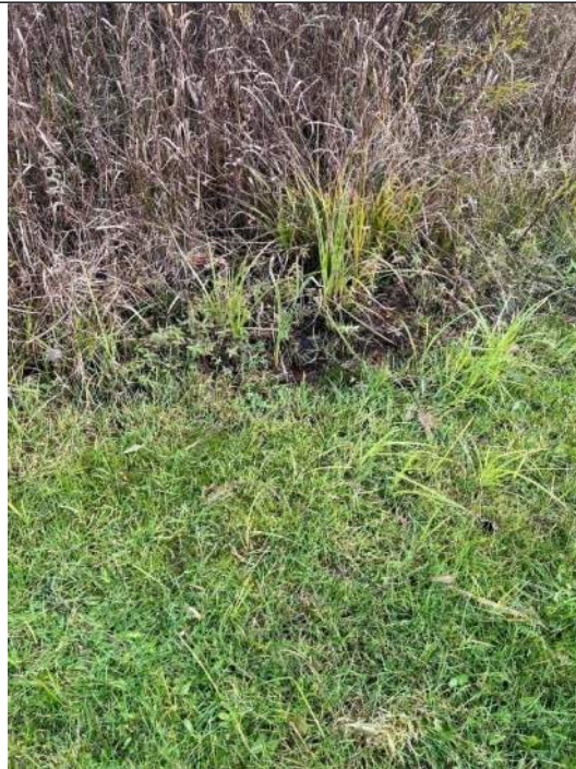
Photo No. 26 – Right Embankment – Downstream Toe Seepage
