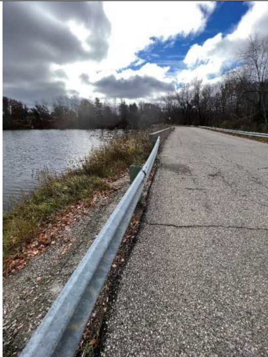
Photo No. 72 – Upstream Side of Left Embankment at Overtopping Section – Looking Left
