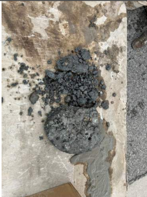
Photo No. 4 – Degraded RCC Layer from B-01
