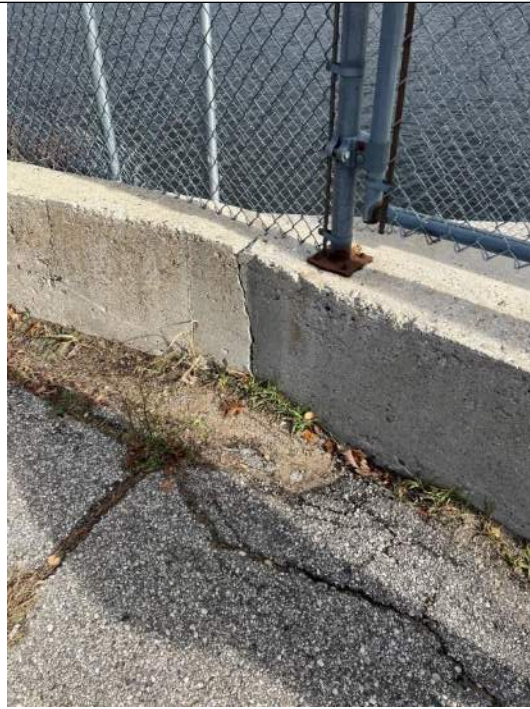
Photo No. 55 – Settlement of Pavement at Upstream Side of Right Primary Spillway Abutment – Looking Upstream
