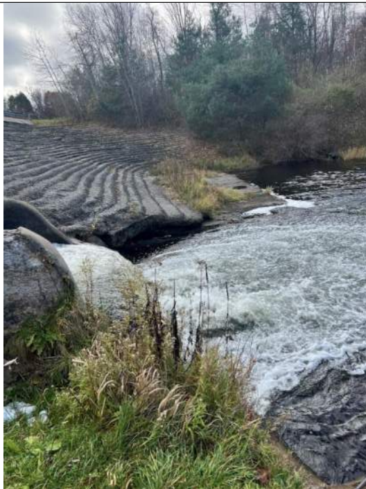
Photo No. 38 – Erosion at Toe of RCC Left Downstream Embankment
