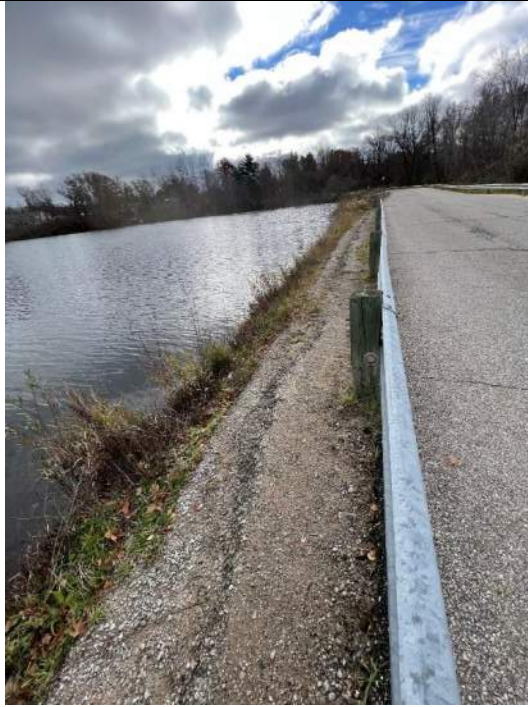
Photo No. 71 – Upstream Side of Left Embankment at Overtopping Section – Looking Left
