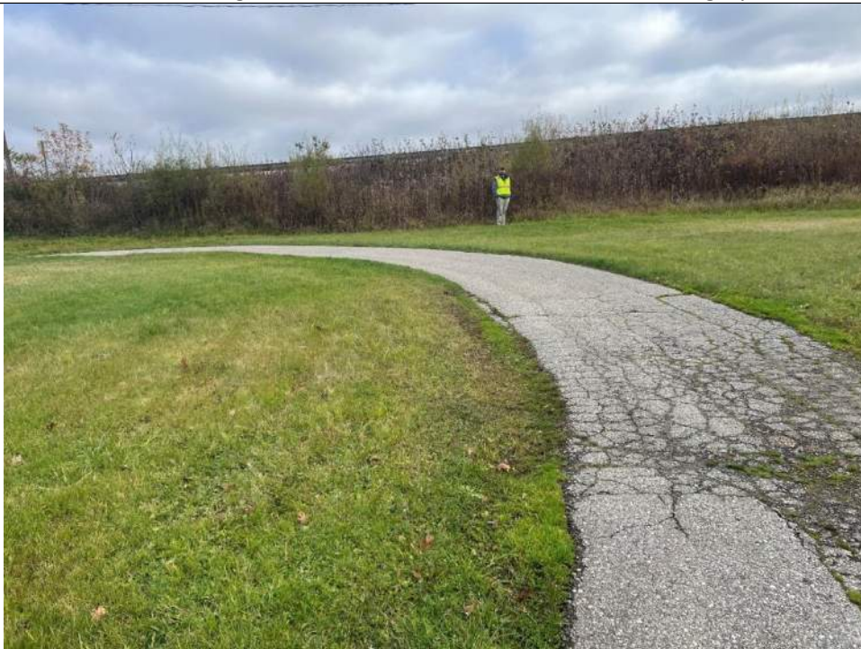
Photo No. 30 – Right Embankment – Downstream Toe Looking Upstream – End of Visible Seepage Right of Primary Spillway
