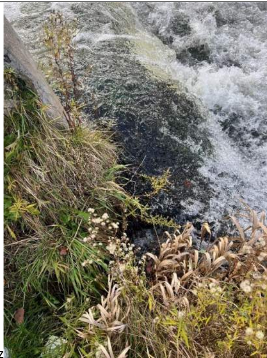
Photo No. 44 – Outlet of Primary Spillway – Erosion at Right Spillway Wall
