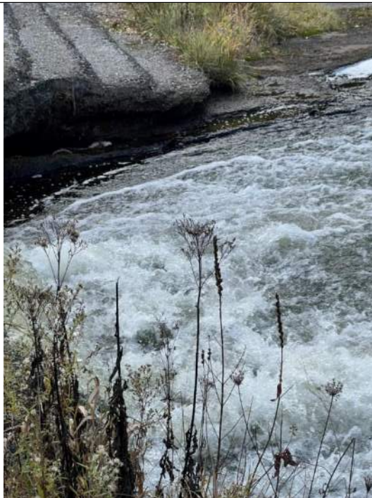
Photo No. 40 – Erosion at Toe of RCC Left Downstream Embankment
