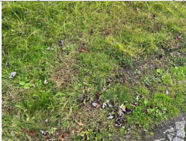
Photo No. 24 – Right Embankment – Downstream Toe Seepage
