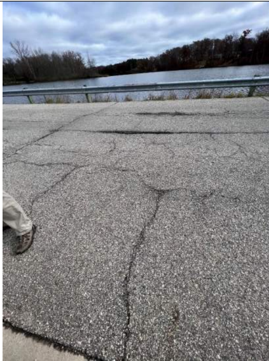
Photo No. 87 – Cracking in Pavement at Crest over RCC – Looking Downstream
