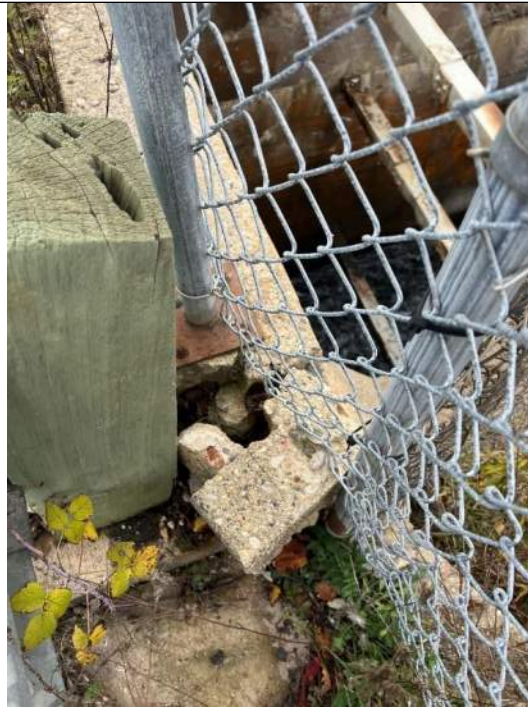
Photo No. 97 – Concrete Deterioration at Right-Side Primary Spillway Downstream Side of Crest – Looking Downstream
