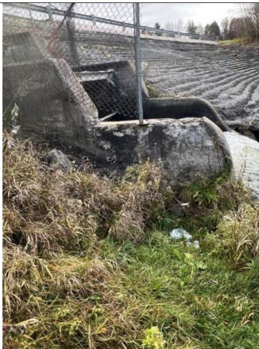
Photo No. 42 – Right Downstream Primary Spillway Wall – Efflorescence and Concrete Deterioration
